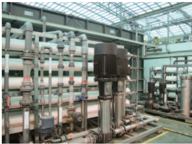
Wastewater Treatment and Reuse System
