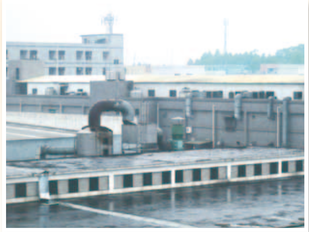
● Central Exhaust System
